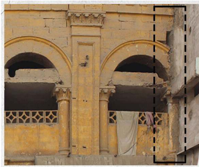
Examining how the encroachments attach themselves to the existing heritage building. This example makes an additional use of a structural beam.
